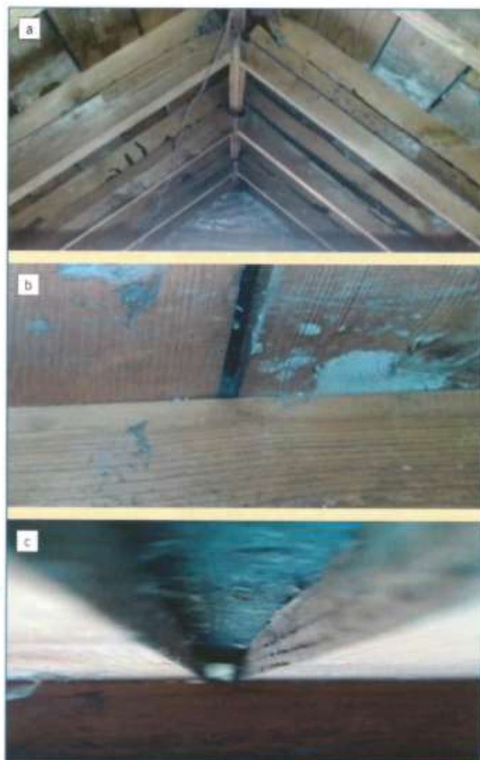
Fig. 1: An example where improved SPF flow could be beneficial at improving gap fill: a) attic ceiling of a 1930's home in Richmond, VA; b) gap formed by the roof deck and roofing truss; c) close up of the gap formed between the roof deck and roof truss
