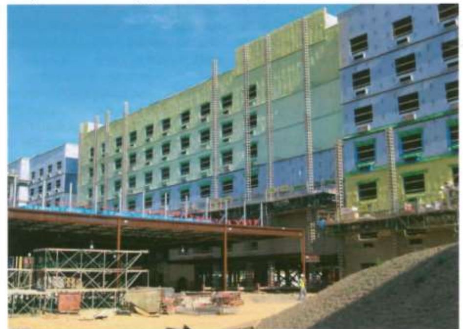
▼ Fig. 3: Closed cell SPF being applied to a hotel in Washington, DC, USA
