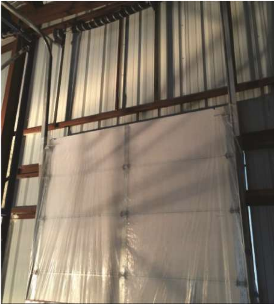
The Keane crew sectioned off designated areas to mitigate overspray damage around the building
