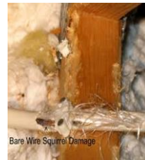
Figure 10 Wires can be fire spots
