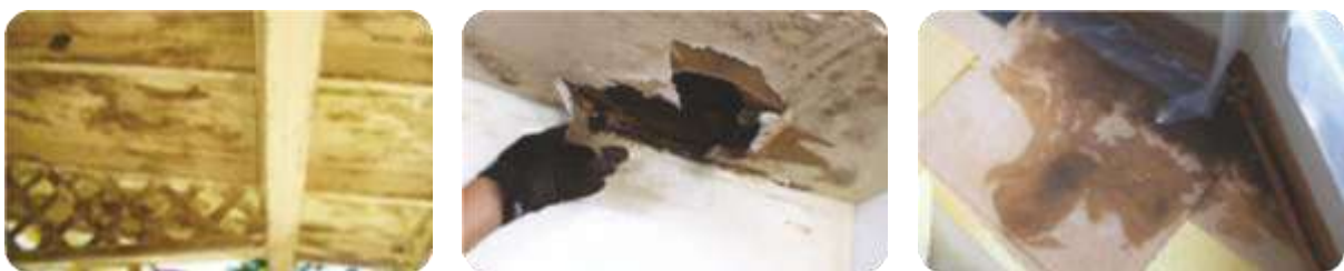
Figure 10 : Moisture is tough saboteur & has to be dealt with firmly
