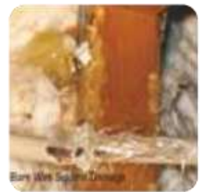
Figure 12 : Wires can be fire spots
