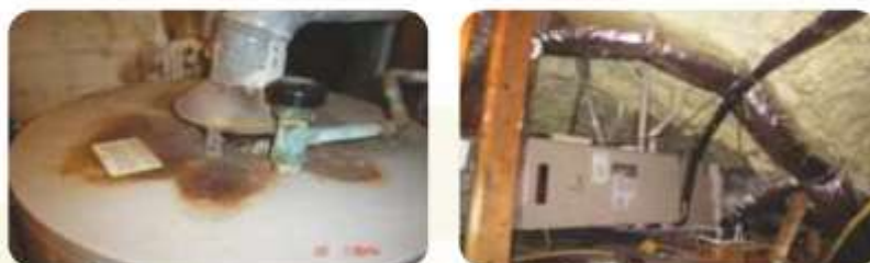
Figure 14 : Open flames inside a sealed space will emit dangerous gases
