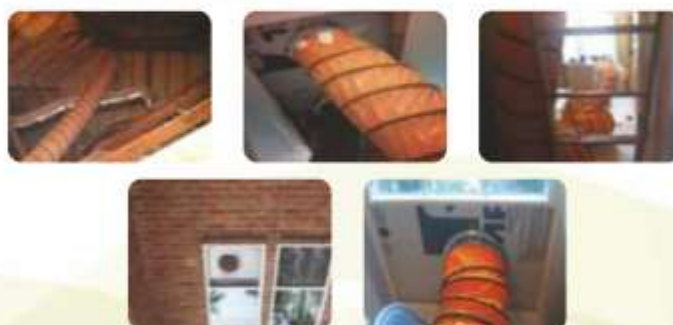
Figure 29 : Local Exhaust Ventilation System
